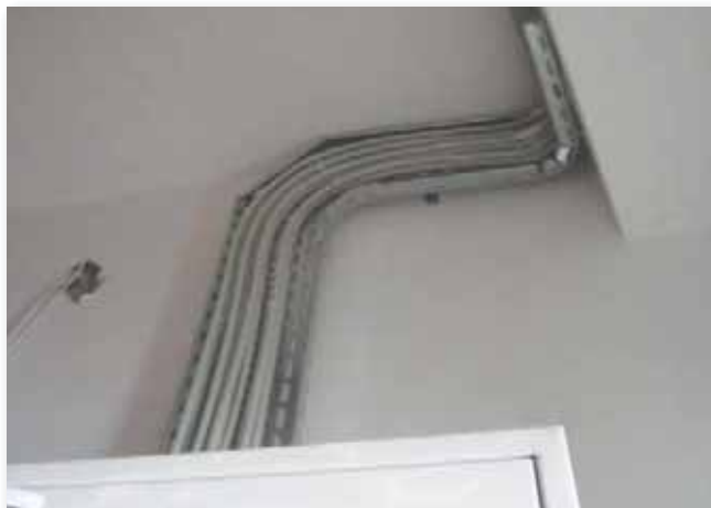
Cables are installed into a single duct in buildings.
