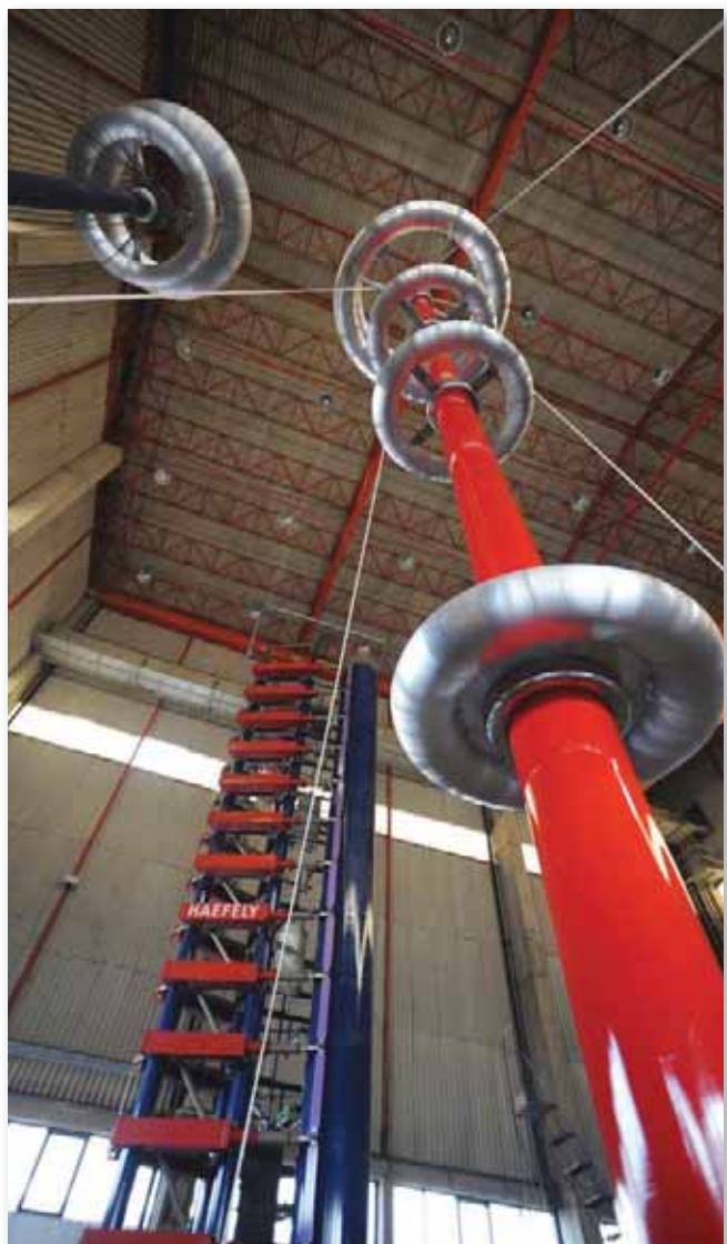
Lightning impulse generator voltage divider.
